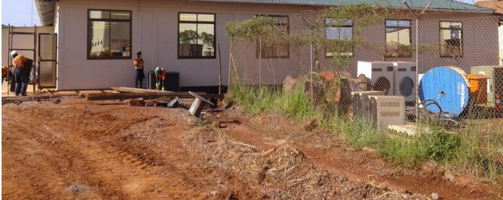
Photos of ongoing Construction of Mess at HME Geita Gold Mine Showing Finishing Works.
