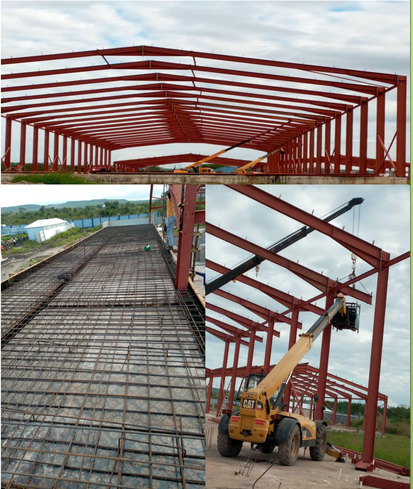
Photos of ongoing Construction of Modern Abattoir at Mpomvu area Geita Council.
