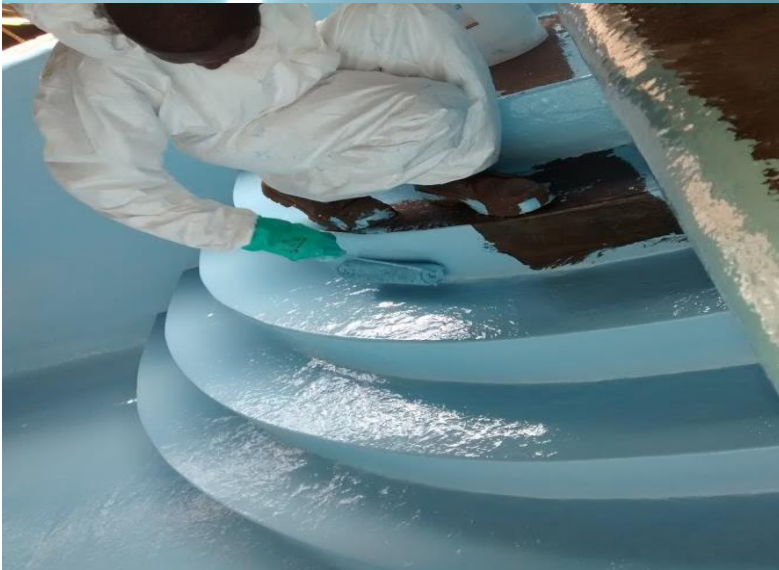
Photos of ongoing Construction of Swimming Pool at Mchauru Village Geita Gold Mine.
