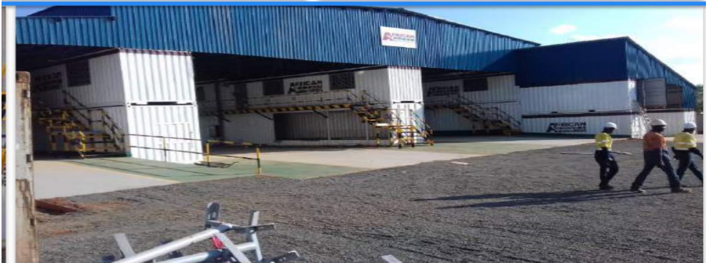
Photos of ongoing Construction of African Underground Mining Service New Complex Office and Workshop
