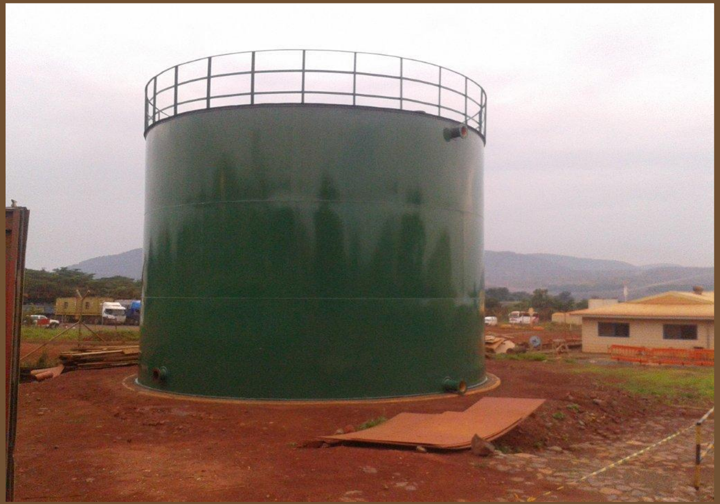
Photos of ongoing fabrication of steel water tank at Geita Gold Mine.
