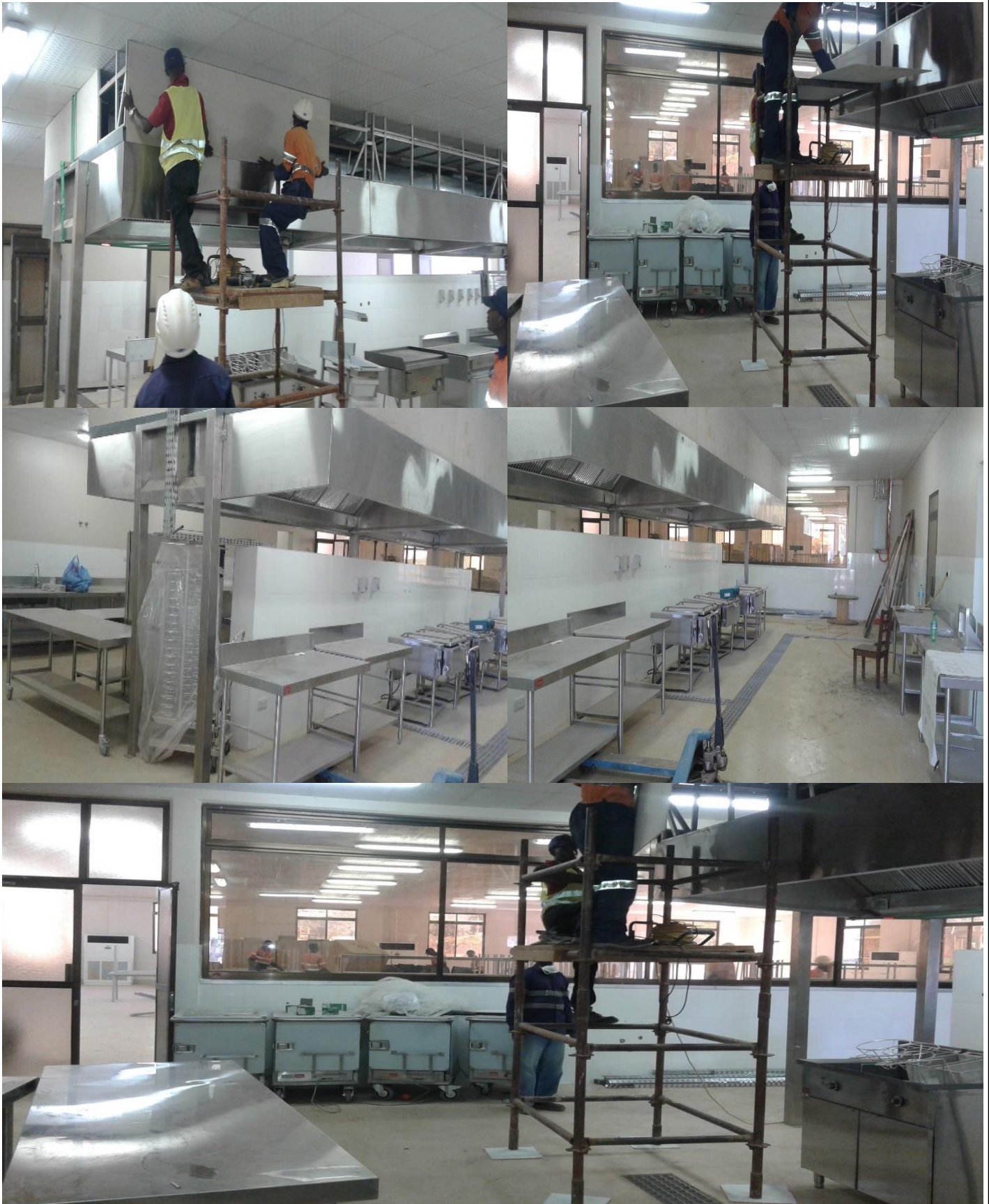
Photos of ongoing Construction of Mess at HME Geita Gold Mine Showing Interior Design Works.
